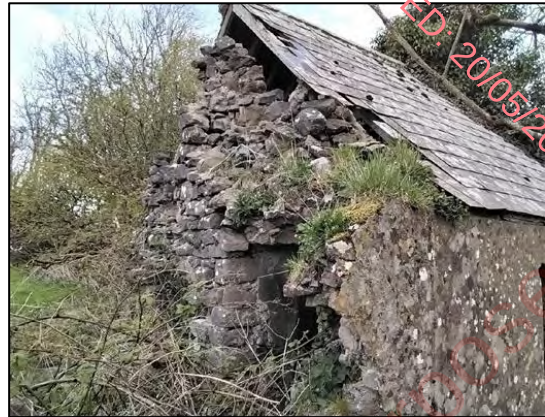
Plate 4-23 External view of the derelict building (Structure 2) showing potential access via open doorway & roof.
