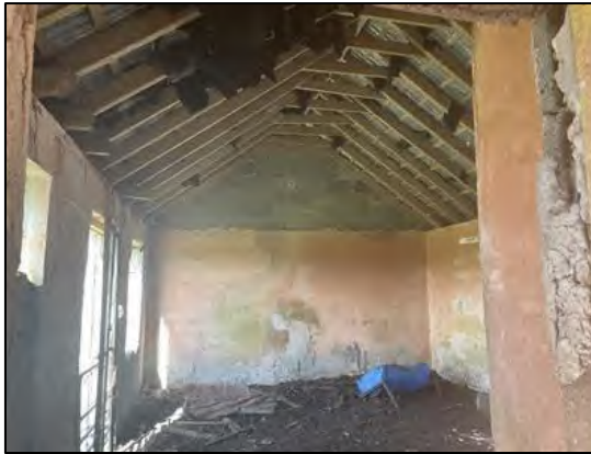
Plate 4-19 Interior view of Structure 1 showing the lack of interior roof lining and exposed nature of the building.
