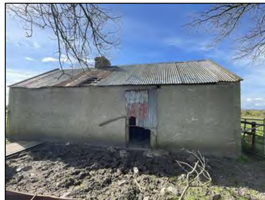
Plate 4-18 North aspect of Structure 1 showing potential access points via the open doorway and gaps under the roof.
