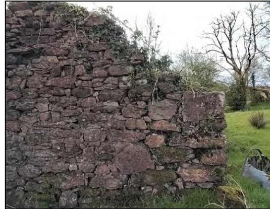
Plate 4-27 Southern wall of associated ruins showing crevices with potential to support roosting bats.
